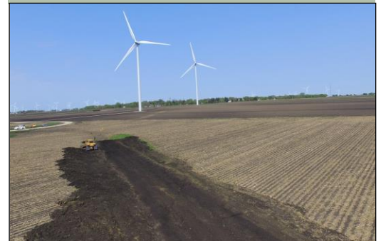
In 2016, a crew builds in the Rose Creek subwatershed of Mower County a grass waterway, one of the practices supported by the federal EQIP
